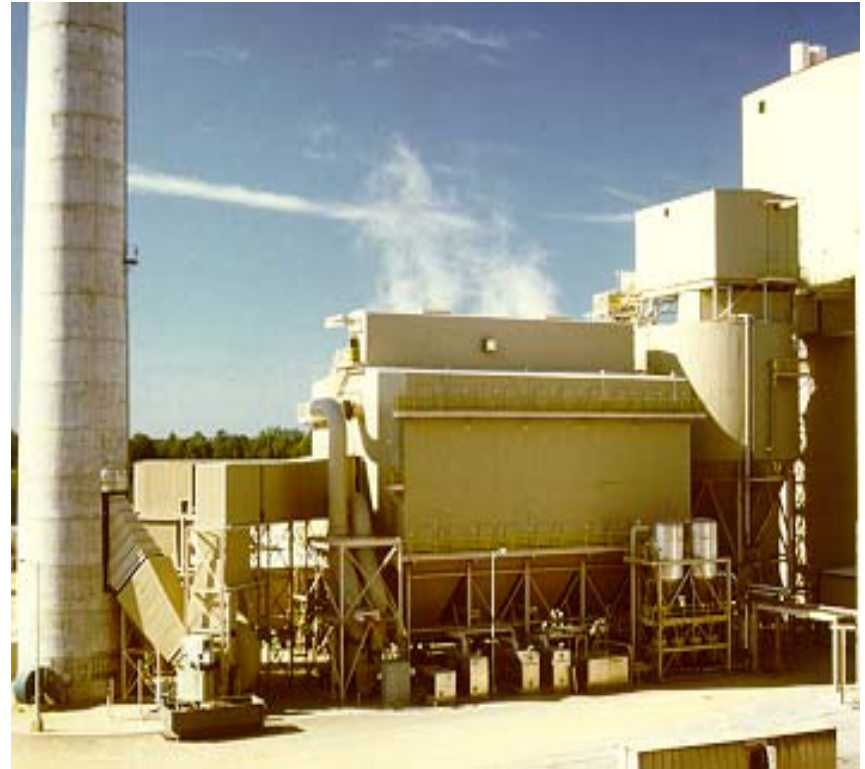
Constellation Power, Inc. Roanoke Valley Unit 1 - 150 MW Roanoke, NC
